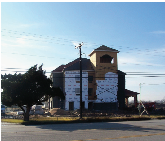
The new La Quinta located on Hwy 35 past Sutherlands is slated to be opened soon.
