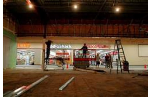
EJ Hersom/Staff Photographer Renovation work continued at the Lilac Mall on Wednesday. The new space will become a Dollar Tree store.
